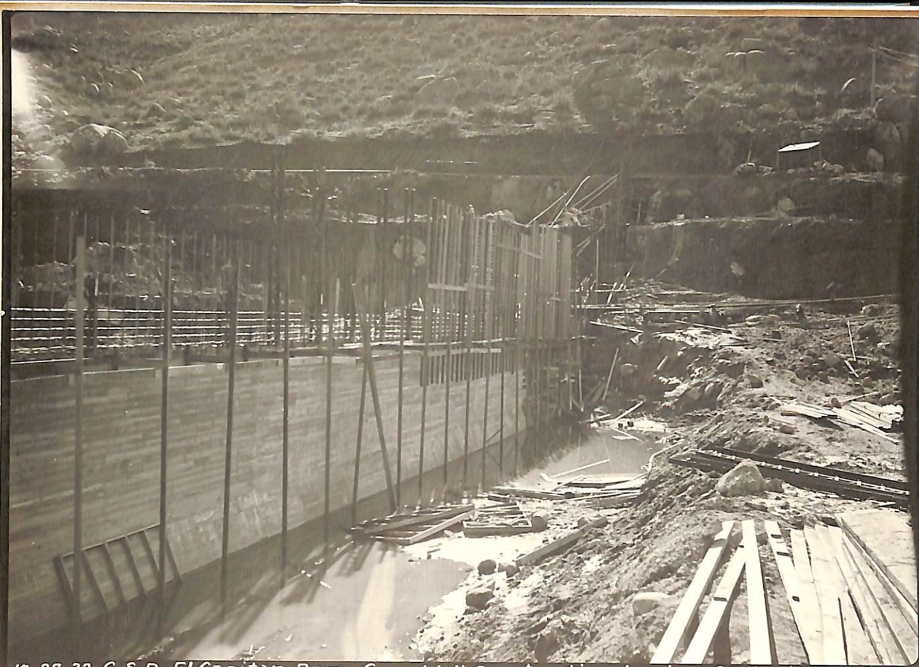
12-27-32. C. S. D. El Capitan Dam. Core Wall Construction, Looking Southerly. EC-233
