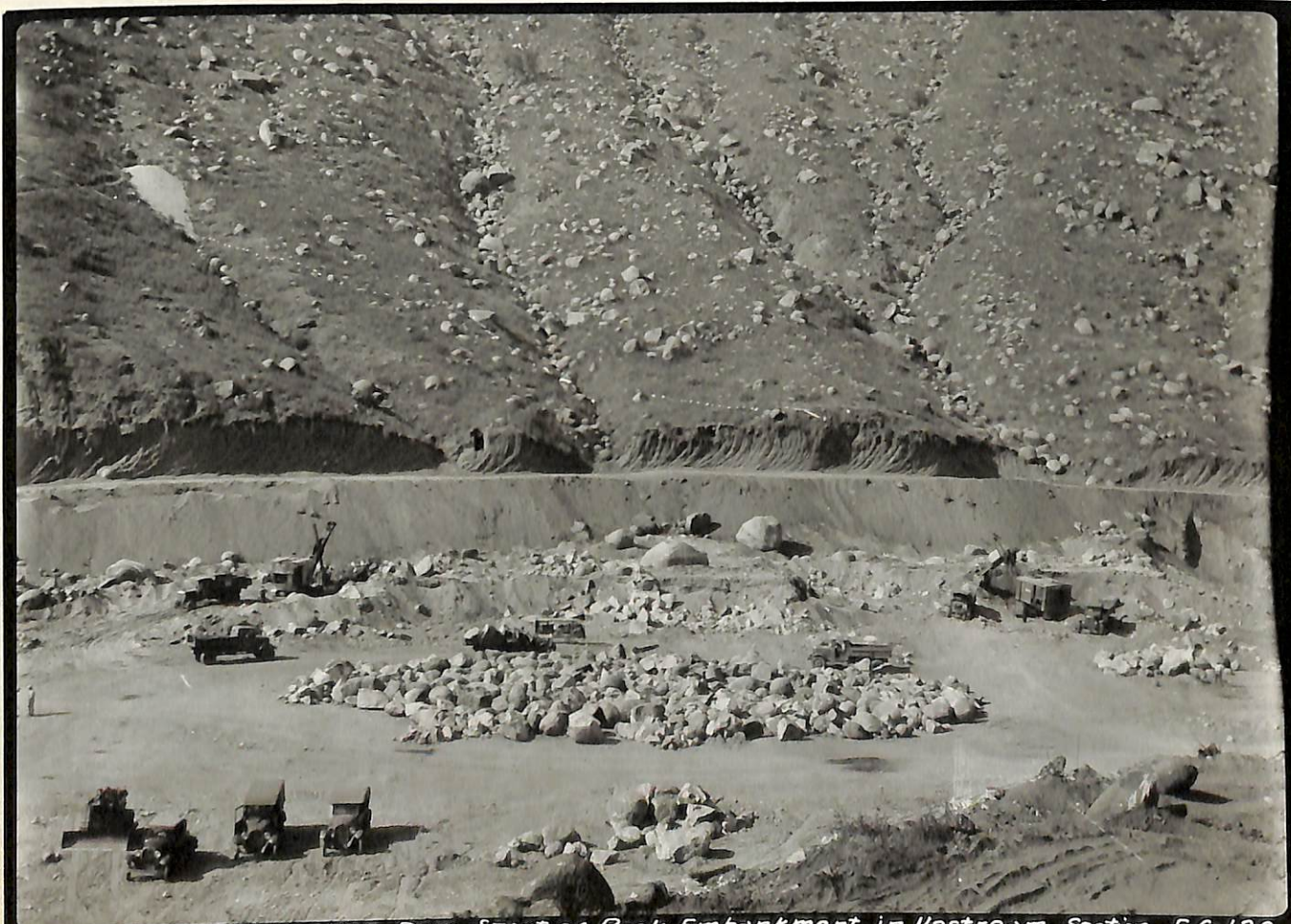
7-25-32. C.S.D. El Capitan Dam. Start of Rock Embankment in Upstream Section. E.G-120.
