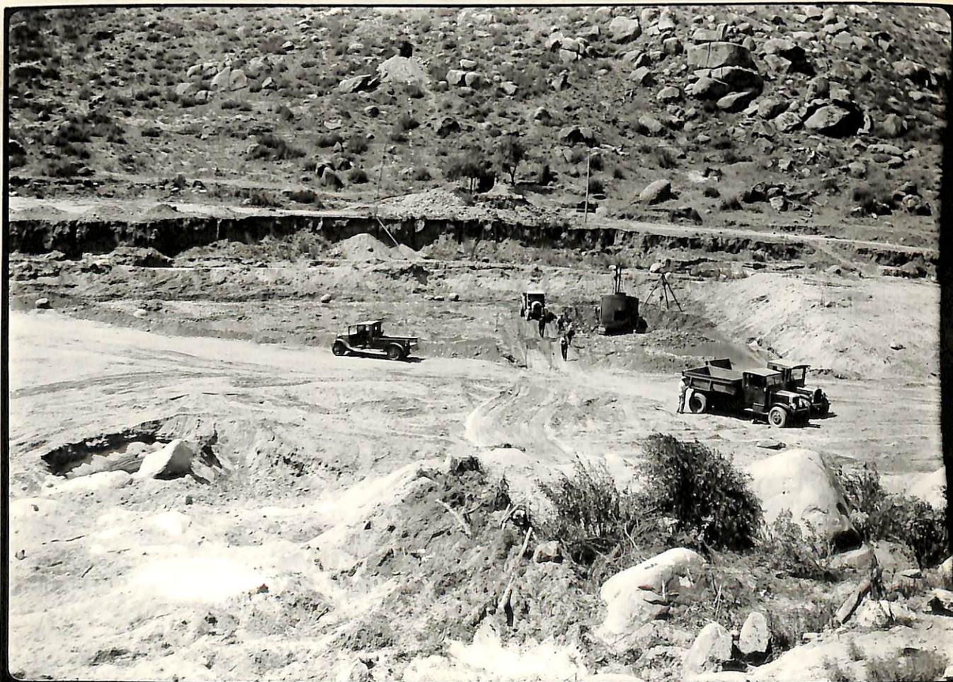
7-1-32. C.S.D. El Capitan Dam. Core Wall and Puddle Core Excavation Looking Southerly. EG-112.
