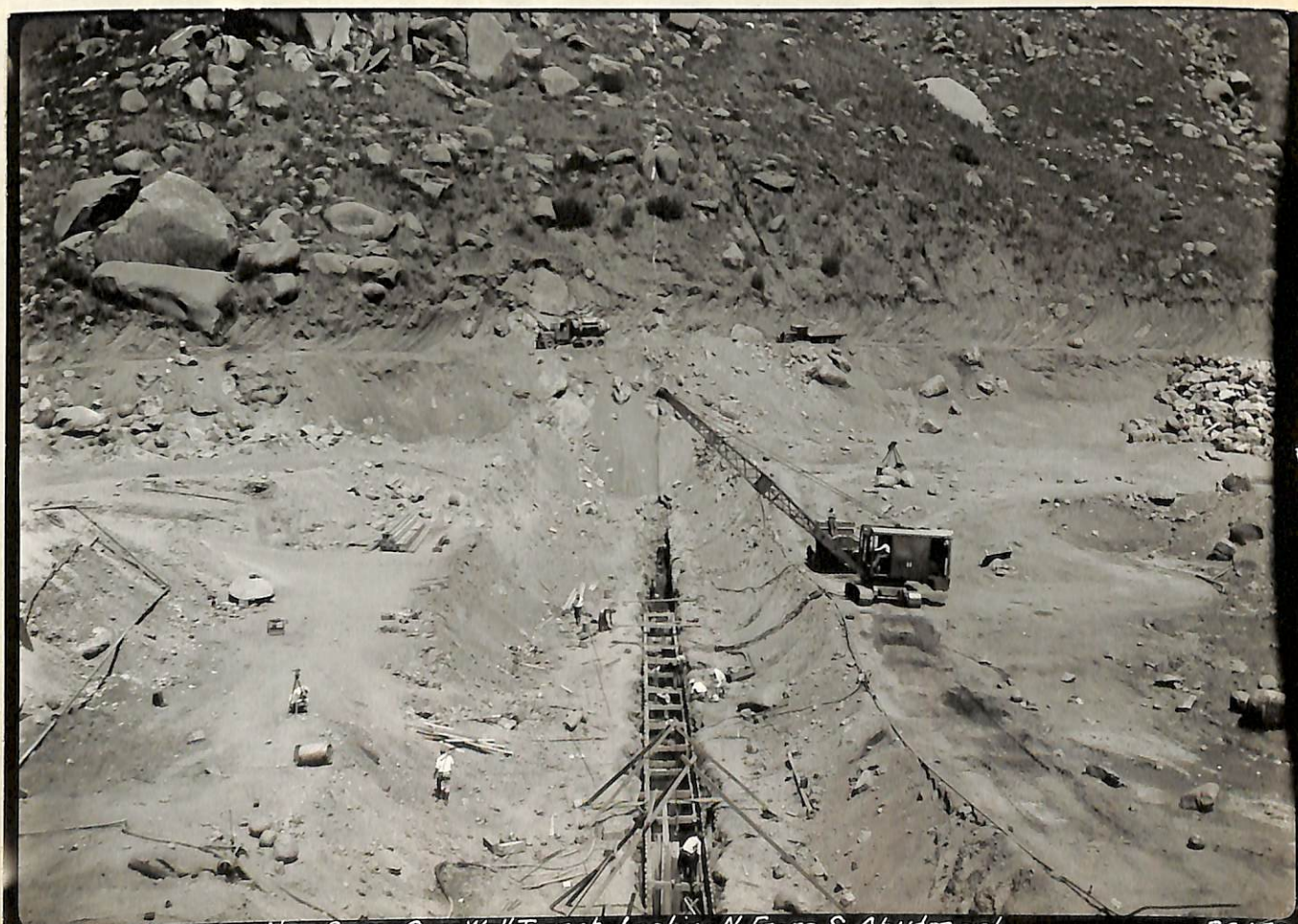
9-9-32 C.S.D. El Capitan Dam - Core Wall Trench. Looking N. From S. Abutment
